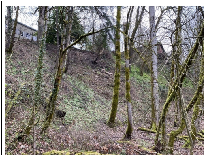
Photo: The steep slope of the Sellwood bluff at the property. The Hearings Officer states that the property “does pose a substantial landslide risk” (page 8) but still recommends the property zoning be changed to more than double the building height and residential density. An example why the recommendation is precarious is the Newell Creek affordable housing project in Oregon City which was built in a landslide zone. Two buildings were subsequently demolished due to landslides, and legal battles ensued 1,2 .
